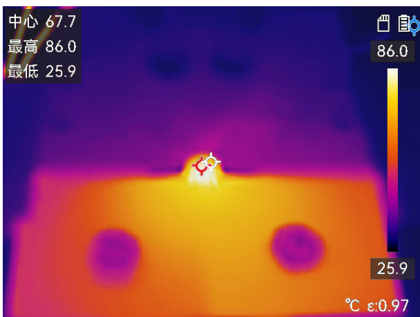
Figure 11. Thermal performance of 40A
